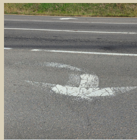
Deficient Pavement Markings and Signage
