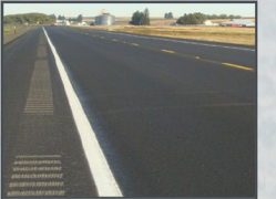
Centerline Rumble Strips
