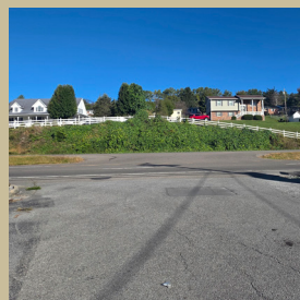
Missing Warning Signs and Advisory Speeds Signs
