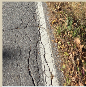
Deficient Pavement Markings and Signage
