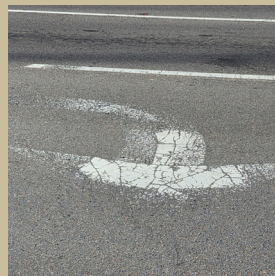
Deficient Pavement Markings and Signage
