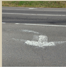
Deficient Pavement Markings and Signage
