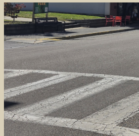
Deficient Pavement Markings and Signage
