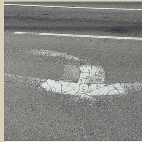
Deficient Pavement Markings and Signage
