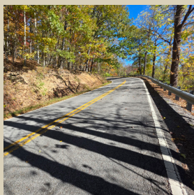
Missing Warning Signs and Advisory Speeds Signs
